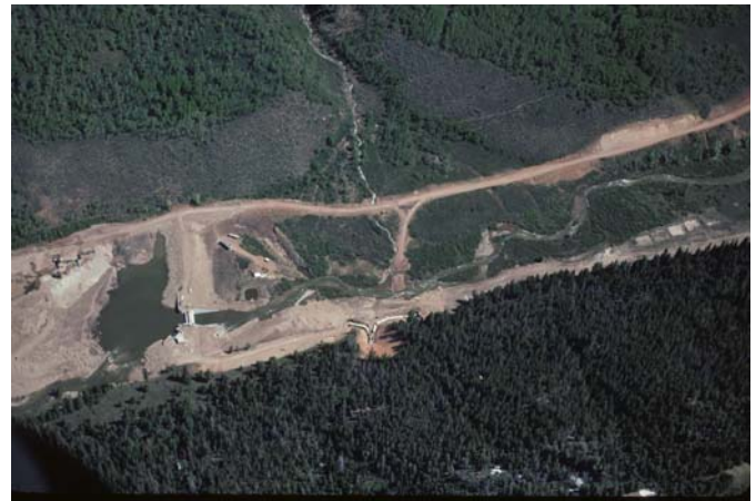
View of the VAT Diversion on the West Fork of the Duchesne River.
